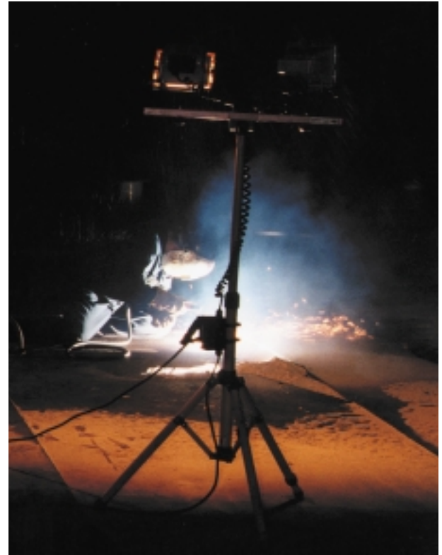
A welding generator's auxiliary power enables this operator to run a bank of flood lights for working in the dark.
