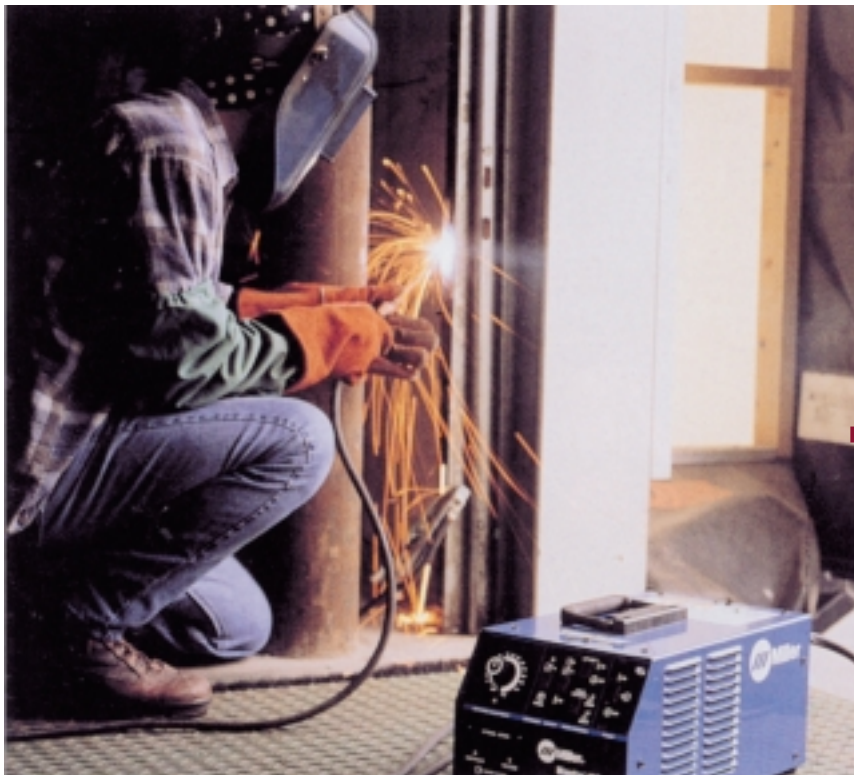
Weight-watching maintenance crews specify inverter-based power supplies for welding to enable welders to easily move around an industrial facility to make timely repairs. Here, an operator shielded-metal-arc welds to repair a garage-door runner. Note how light he travels — just the power supply, electrode, and electrode holder.
